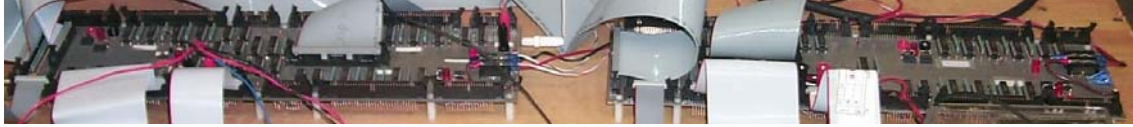
Figure 5: The switch boards primarily provide power switching and I/O routing to and from each of the arms of the burn-in stand. Each board can handle up to eight arms of eight hybrids. They are further described in section 2.4.
